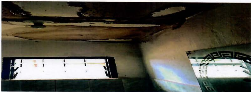
GAC photo 1: Renovated PIU Office located in Robertsport, Grand Cape Mount, Abandoned and out of use
