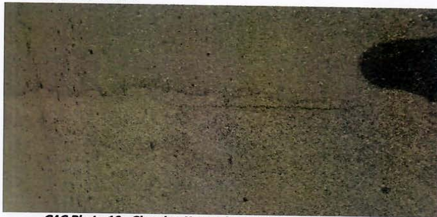
GAC Photo 10: Showing Unrepaired Crack on Asphalt along the Gbarnga to Ganta-Guinea Border road corridor in Lot 2
