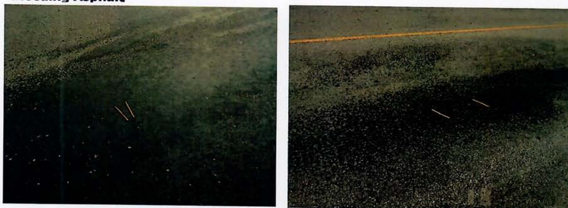
GAC Photos 3 Showing Bleeding Asphalt on Pavement Surface, Monrovia to Gbarnga corridor in Lot 1
