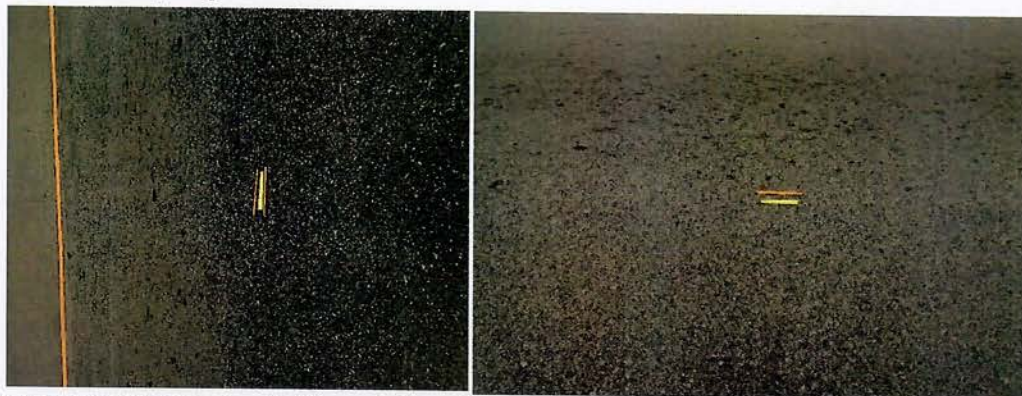
GAC Photos 8: Showing Settlement along the road corridor from Gharnga to Ganta Guinea Border
