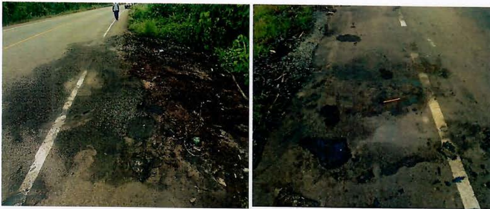
GAC Photo 4 Showing Damage to Asphalt at 138+500 km LHS
