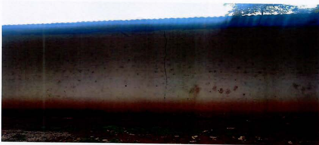
GAC Photo 6b: Showing damage to building and crack to wall of building in Vaitekeh Village
