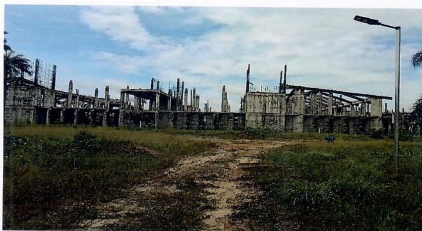
Partial view of the uncompleted construction work at the New Redemption Hospital located in Caldwell
