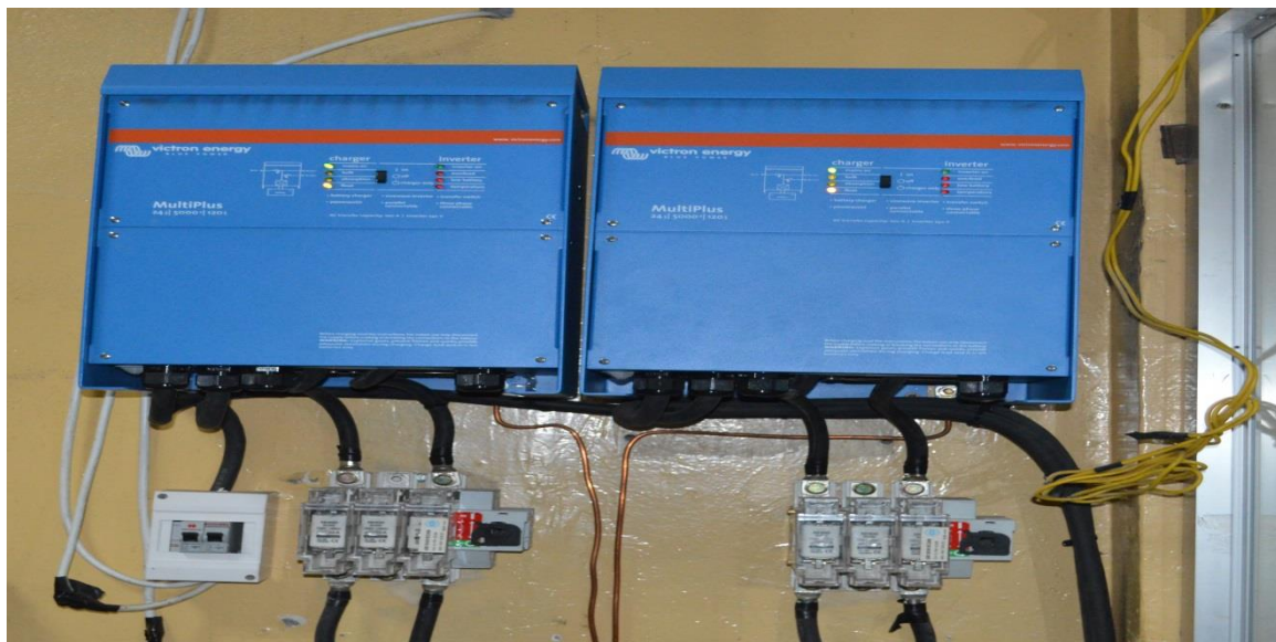
Figure 8: Battery Bank System
