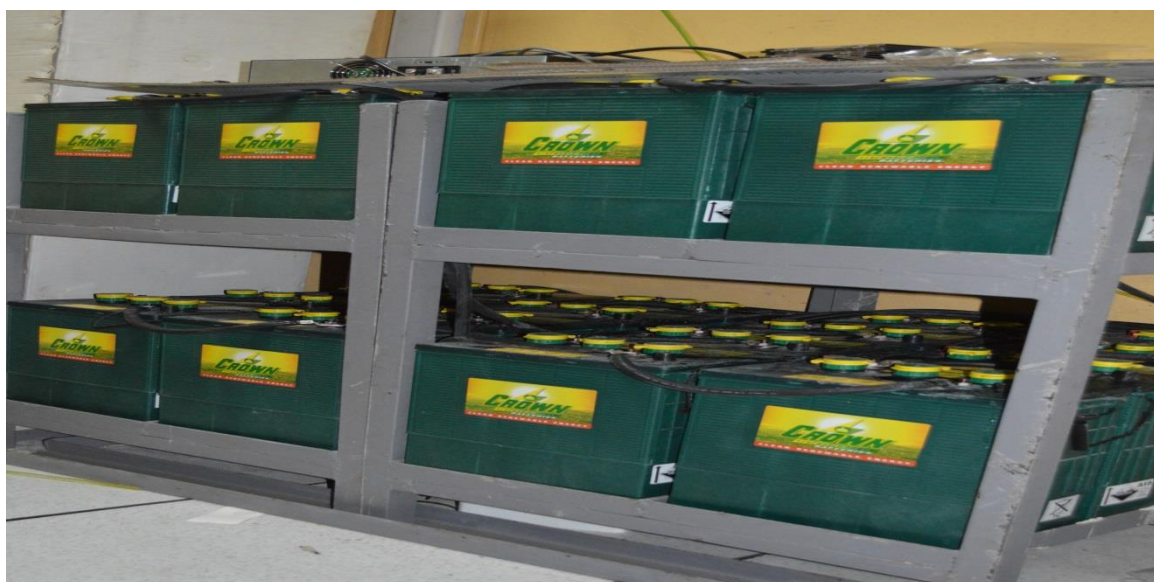
Figure 9: Battery Bank System
