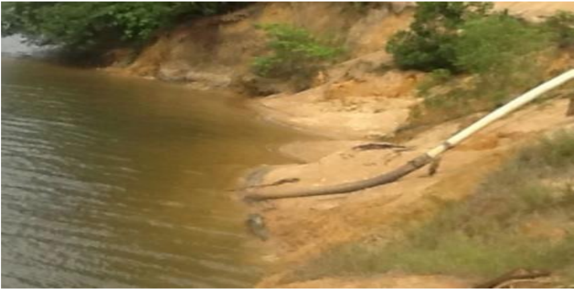
Source: GAC Photo 7, River Bank Caving In St. Paul
