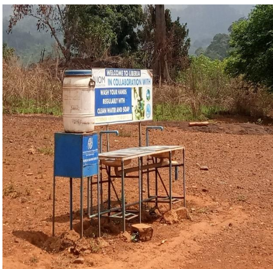
Non-functional hand washing station at Yekepa land border
