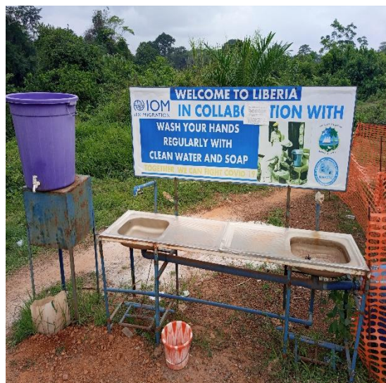
Non-functional hand washing station at Ganta land border
