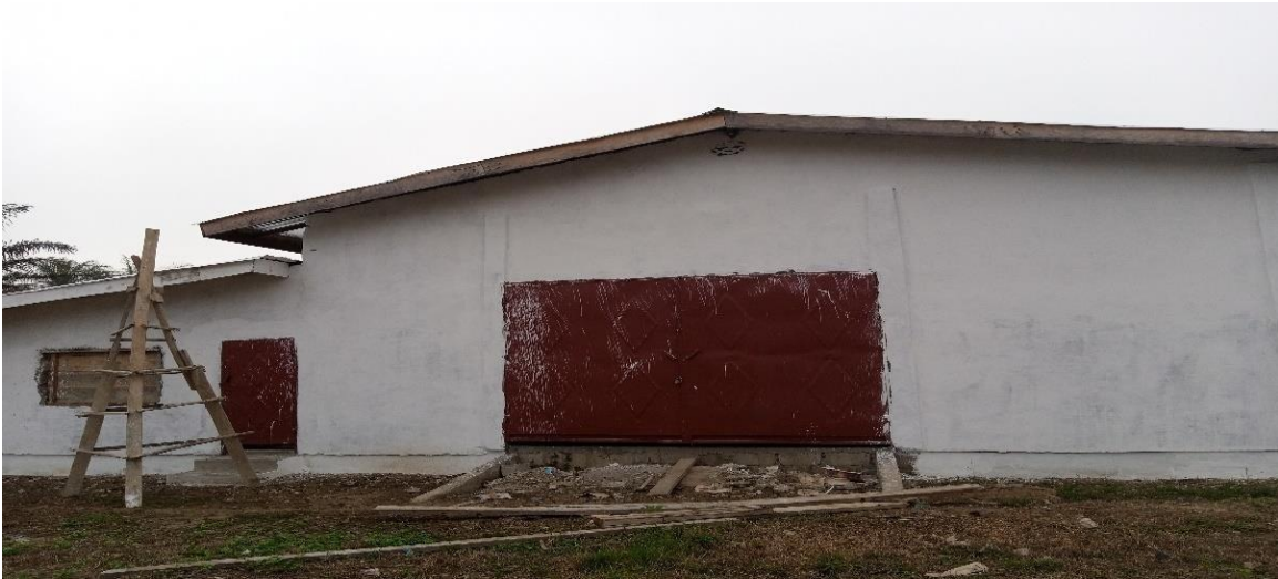
Front View of the Incomplete Warehouse in Karnwee, Saclepea Mah
