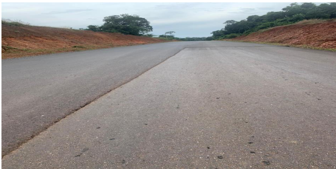
GAC Photo: partial view of the 10.246km out of 80km of wearing course completed by the contractor
