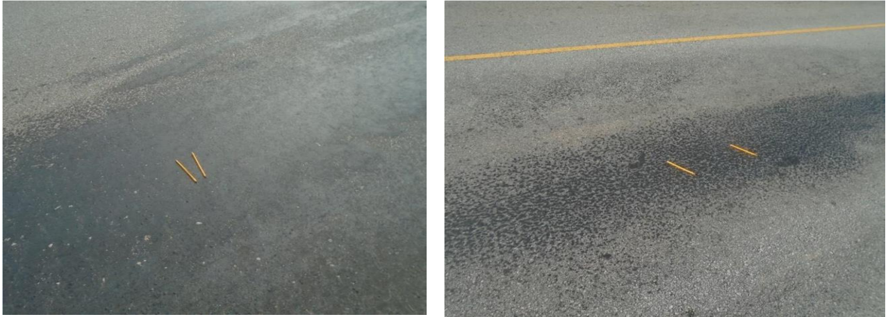
GAC Photo 3: Showing Bleeding Asphalt on Pavement Surface, Monrovia to Gbarnga corridor in Lot 1
