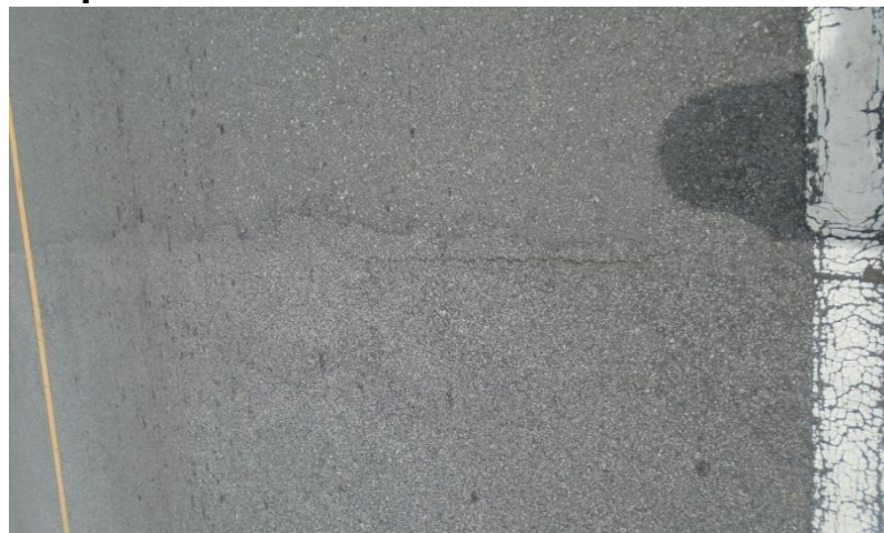
GAC Photo 11: Showing Unrepaired Crack on Asphalt along the Gbarnga to Ganta-Guinea Border road corridor in Lot 2
