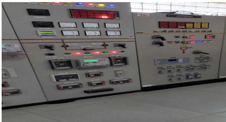
GAC photo: Control Units in Kakata Substation
