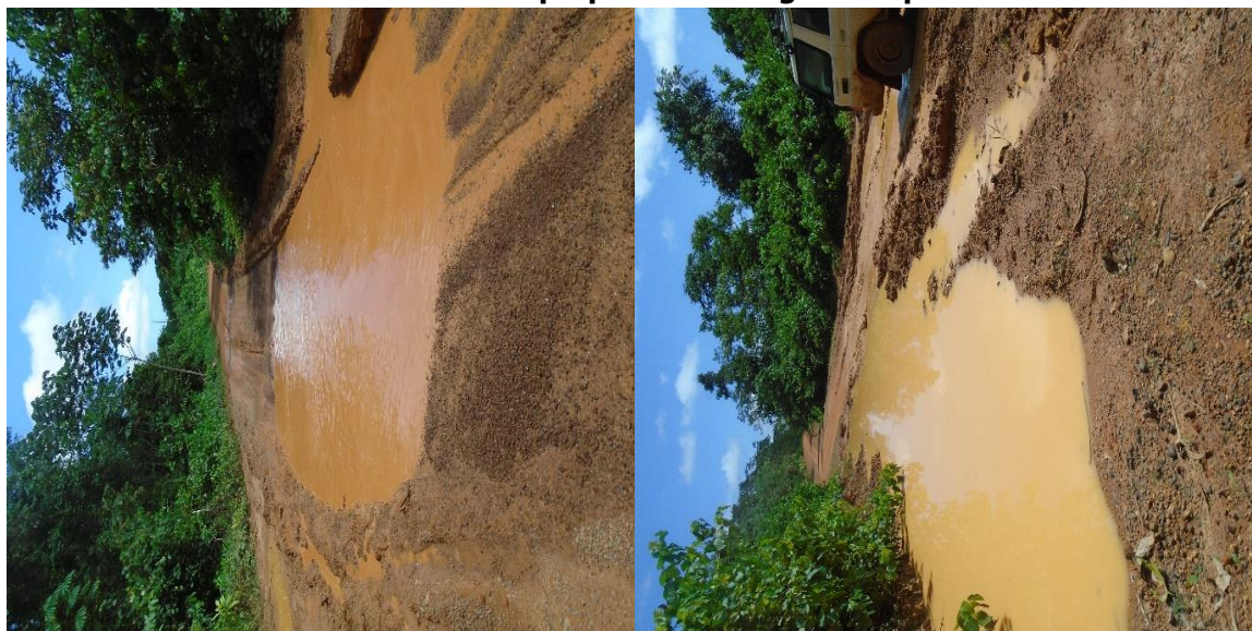
GAC Photos 3 showing improper backfilling, compaction and gabion work on ITI to Greenville Road Project
