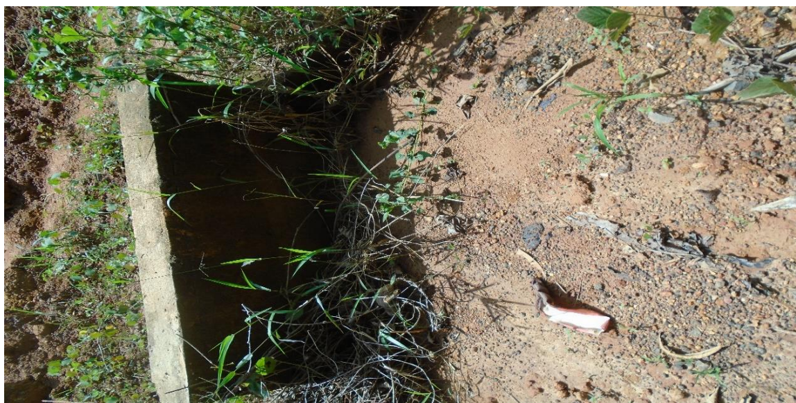
GAC Photos 3 showing blockage of the RCP on ITI Bridge to Greenville 130km, Sinoe County Road project
