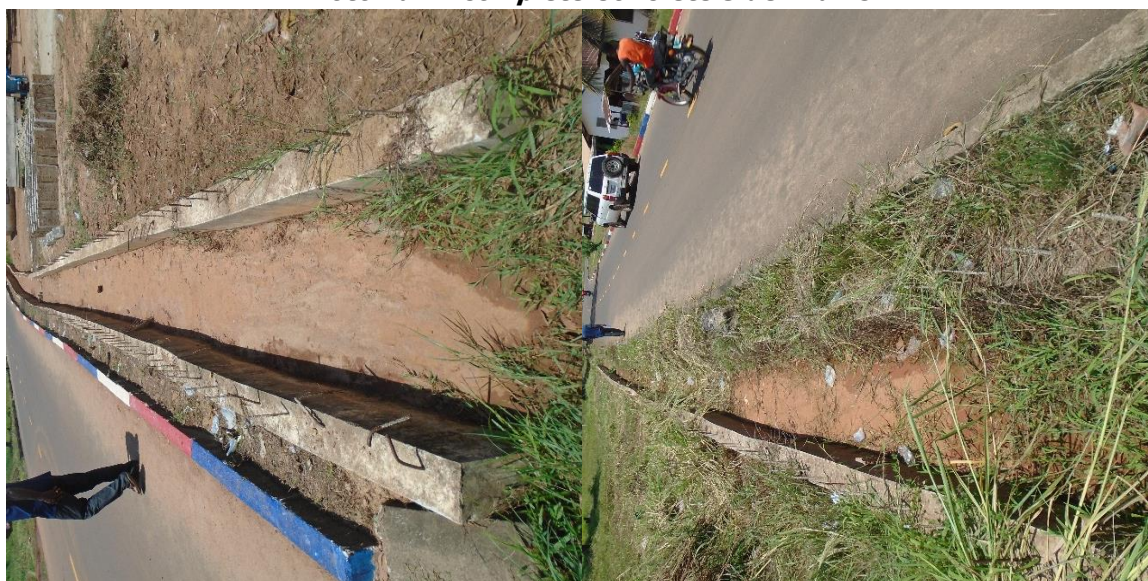
GAC Photo 1a showing incomplete concrete side drains that yet to receive concrete slabs/covers on the carriage way of Buchanan Fair Ground
