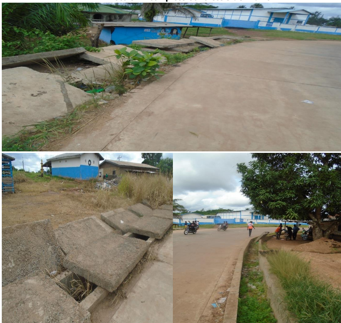
GAC Photo 8 showing incomplete concrete side drains that yet to receive concrete slabs/covers on the Gbarnga Broad Street.
