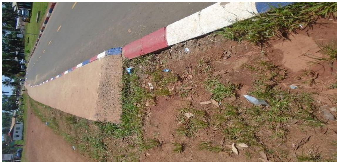
GAC Photo 1b showing incomplete concrete sidewalks and curbs on the carriage way of Buchanan Fair Ground
