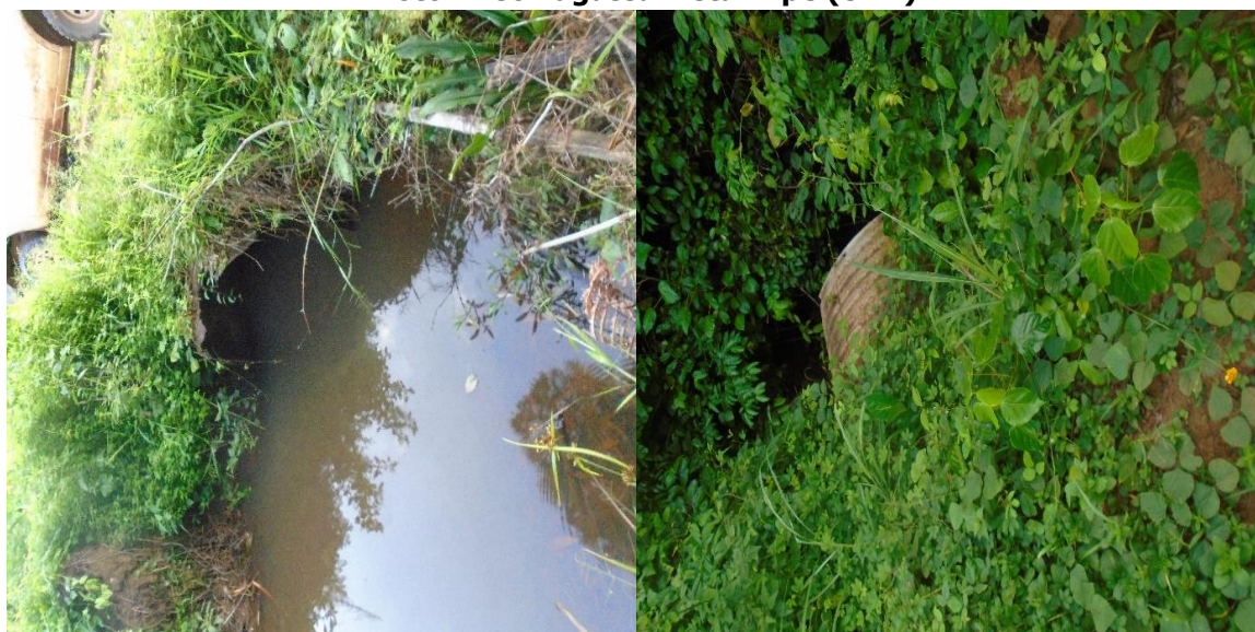
GAC Photos 7 showing CMPs on the carriageway of Zekepa to Tappita Road in Nimba County
