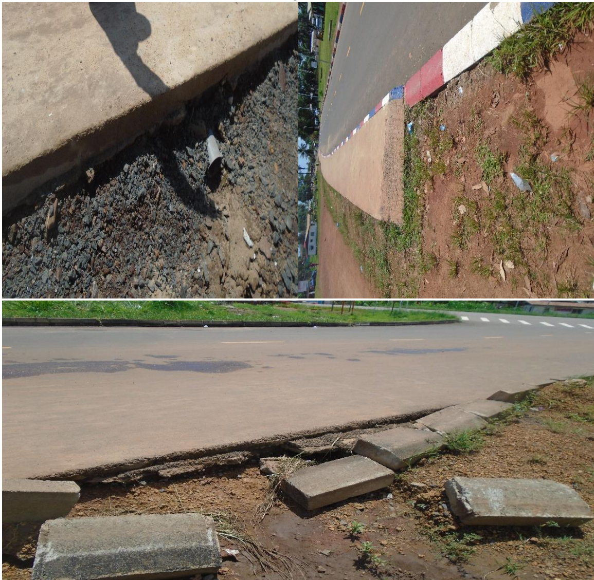
Photo 1b: Incomplete Concrete Sidewalks
