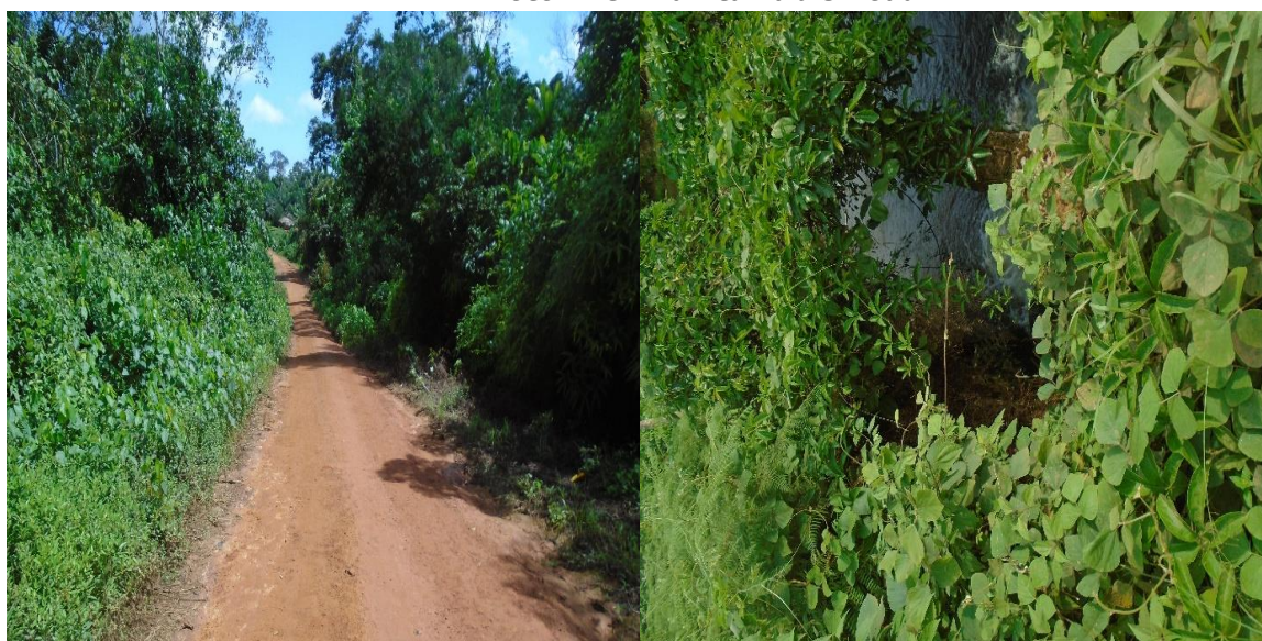
GAC Photos 2 showing road that has not yet received clearing, grubbing, laterite (proper gravel layer) works on Buchanan to ITI Bridge to Cestos City
