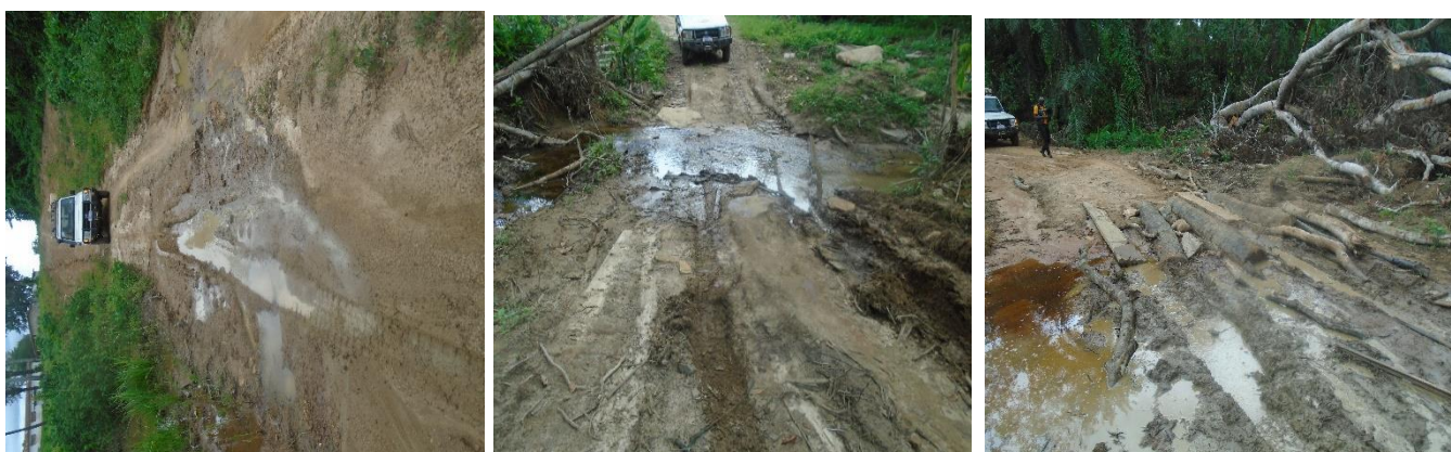
GAC Photo 5a showing improper earthwork and drainage work on the carriage way of Garyea to Gbanlata Road Project
