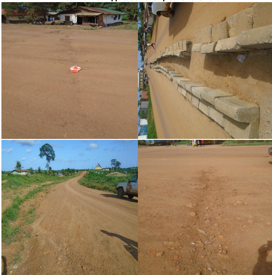
GAC Photos 6 showing Non-Application of Chip Seals Pavement in Greenville Barclayville cities respectively
