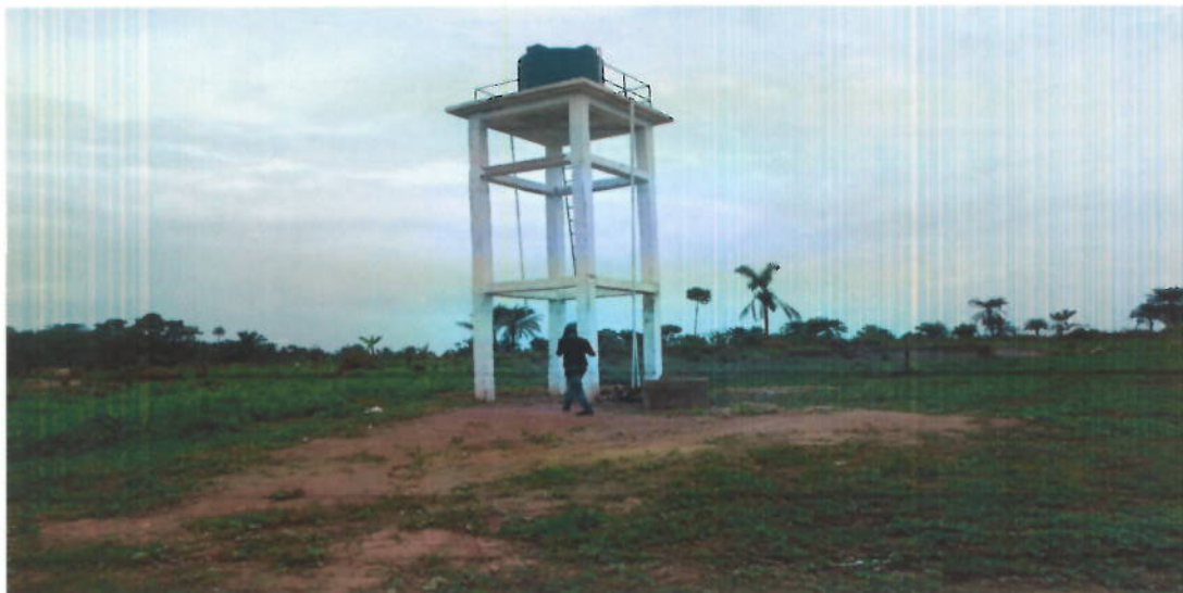
Foya Water Tower - No Connection
