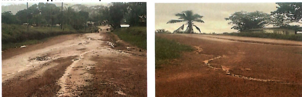
GAC Picture 2 showing Non-Application of Chip Seals Pavement in Bopolu City
