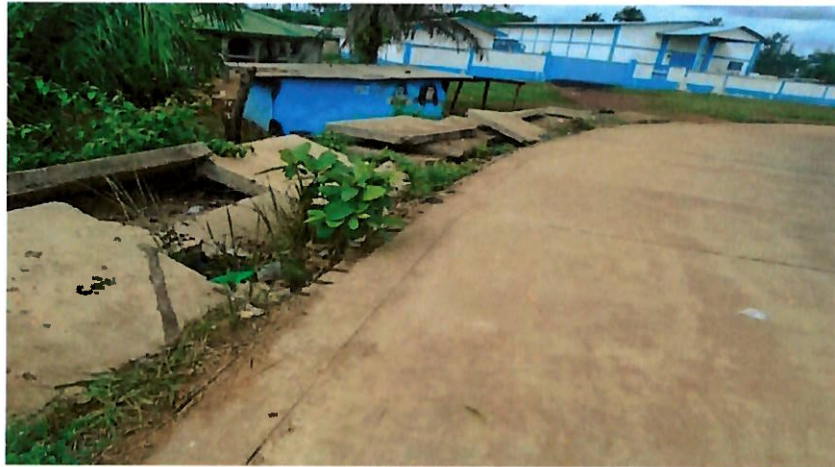
Photo 11: Incomplete Concrete Side Drains
