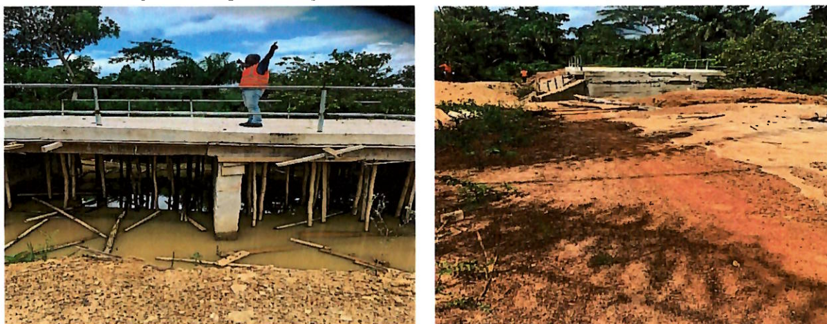
GAC Picture 9 showing the incomplete and uncompacted Bridge on Zorgowee-Dulay Road
