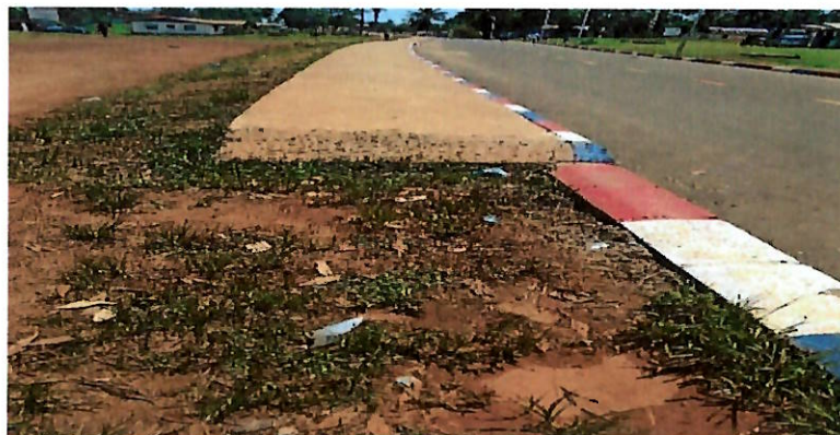
GAC Picture 7 showing incomplete concrete sidewalks and curbs on the carriage way of Buchanan Fair Ground
