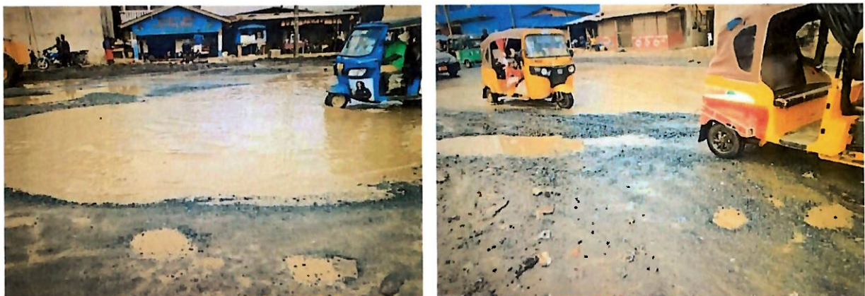
Photo 1: Contractor Abandonment of Urban Paved Road Project (Johnson Street Bridge to St. Paul Bridge Road corridor - GAC Picture1: showing incomplete asphalt overlay on the carriageway from Johnson Street to St. Paul Bridge
