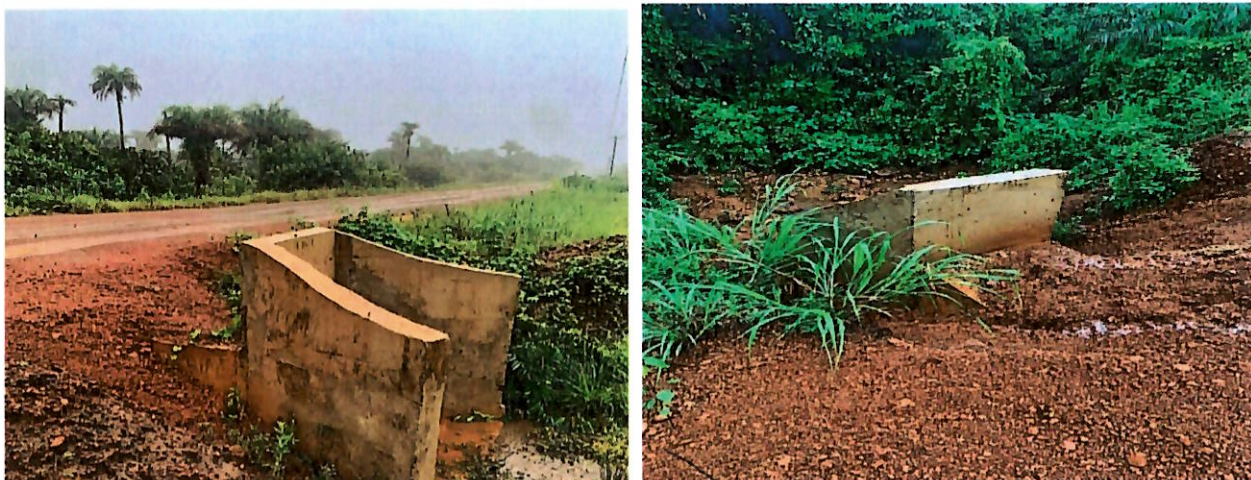
GAC Picture 5 showing unpaved asphalt road and improper compaction of curbs along the Madina Junction to Robertsport
