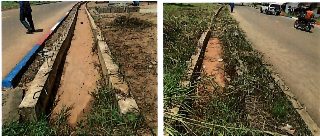
GAC Photo 6 showing incomplete concrete side drains that yet to receive concrete slabs/covers on the carriage way of Buchanan Fair Ground
