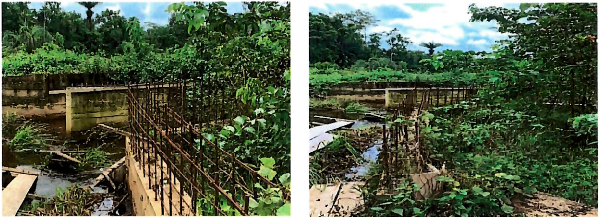
GAC Picture 8 Showing an Incomplete and Abandoned Bridge on Kolilia-Palila Road Corridor, Bong County
