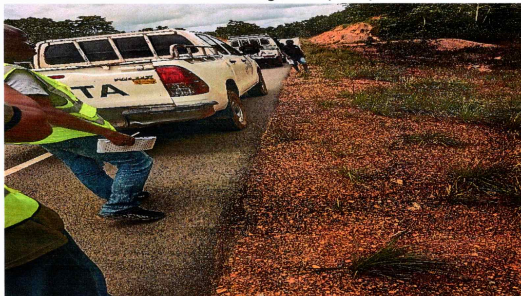
GAC Picture 6: Showing incomplete side drains and guardrail along the 61km road corridor
