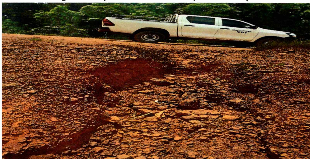
GAC Photo 3: Showing non-compliance with contract specifications (erosion around RCPs)
