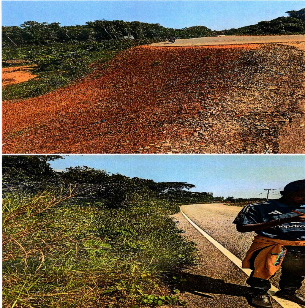
GAC Photo 4: Showing overhanging tree, vegetation, and lack of guardrail along Ganta to Saglepie in Lot 1 (39km)
