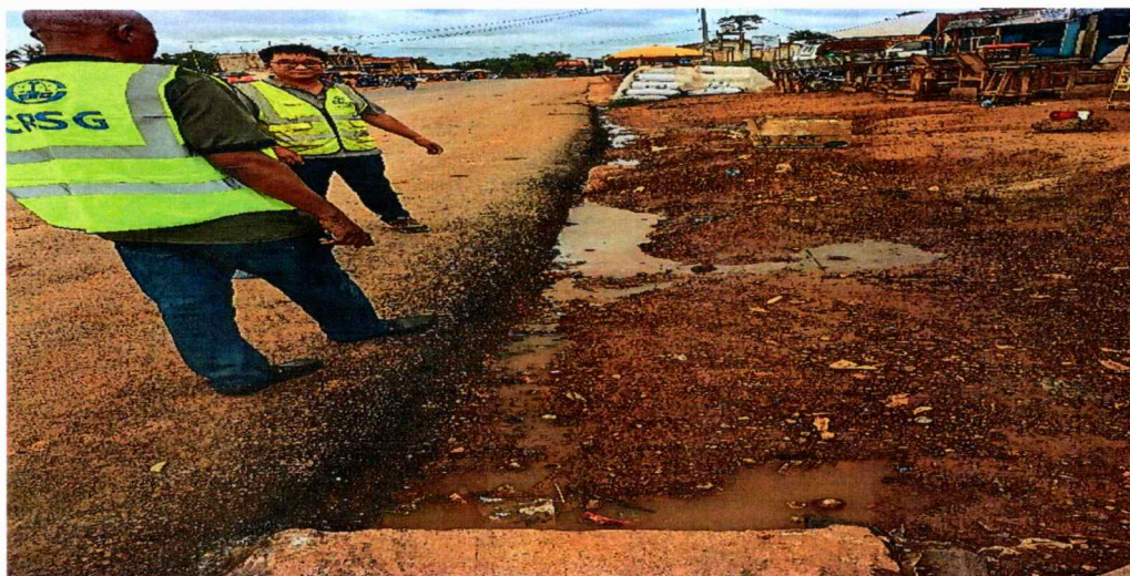
GAC Picture 5: Showing incomplete side drains along the 61km road corridor
