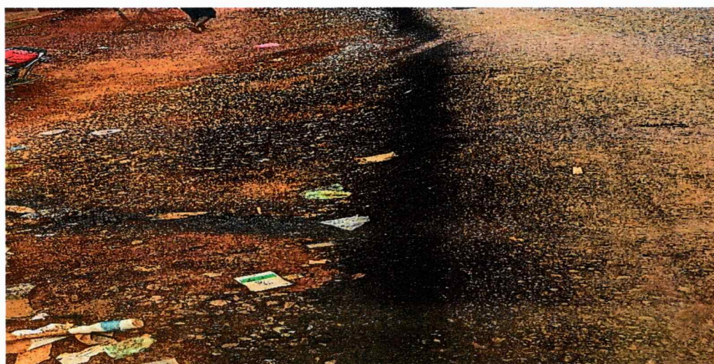
GAC Picture 4a: Showing Road verges unsupported, cracking and breaking
