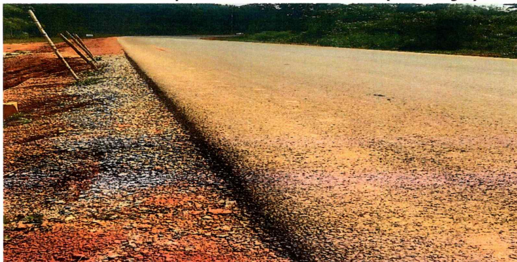
Photo 4a: Non-Compliance of Rehabilitation Works (Road Verges)
