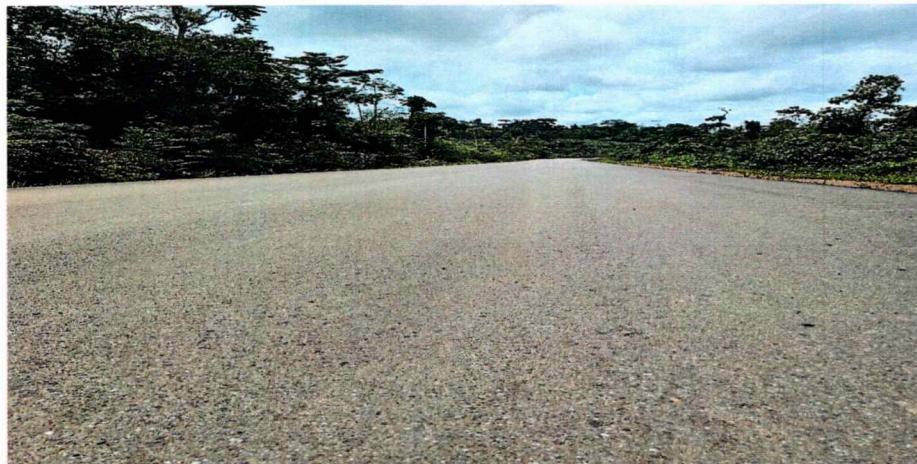
GAC Photo: partial view of the Fishtown to Kilepo road- 20km, uncompleted
