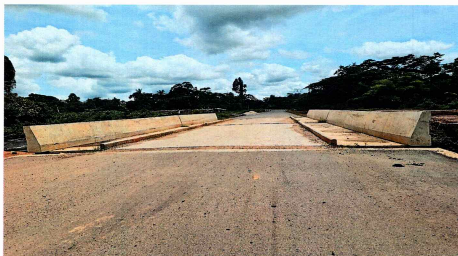
GAC Photo: Partial view of the bridge #1 (30 meters)- Fish Town to Kelipo Road, Uncompleted
