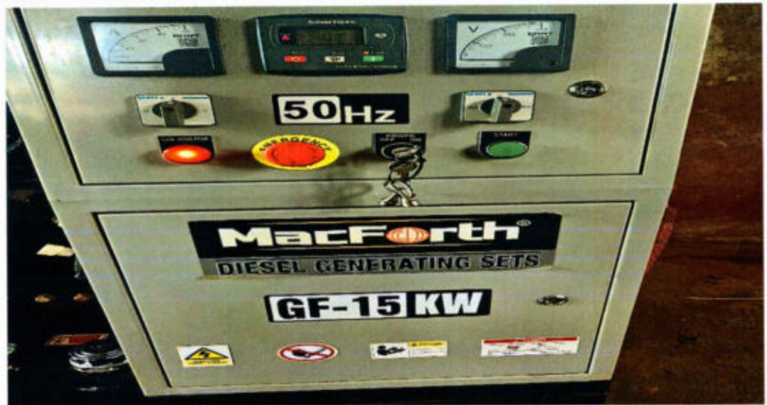
Picture 1: 15KVA Macforth MF Generator
