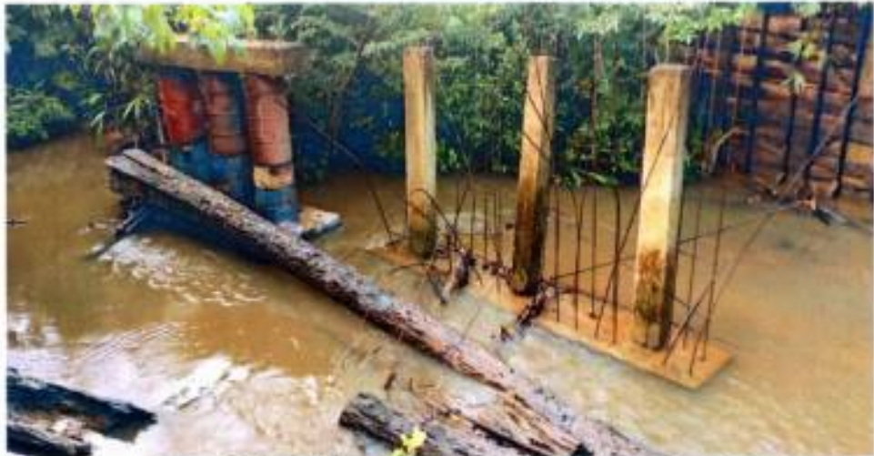
Construction of Whoo Bridge, - Cost US$50,006.00, Dorpa Town, Dist. #9, Contractor: Atlantic Engineering and Construction Company Limited
