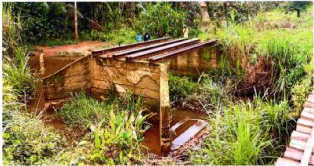
Construction of Bridges Cost US$20,000.00 in Yarmein and Gbehlageh in District No. 3: (New Yekepa); Contractor: LIDA Liberia Limited
