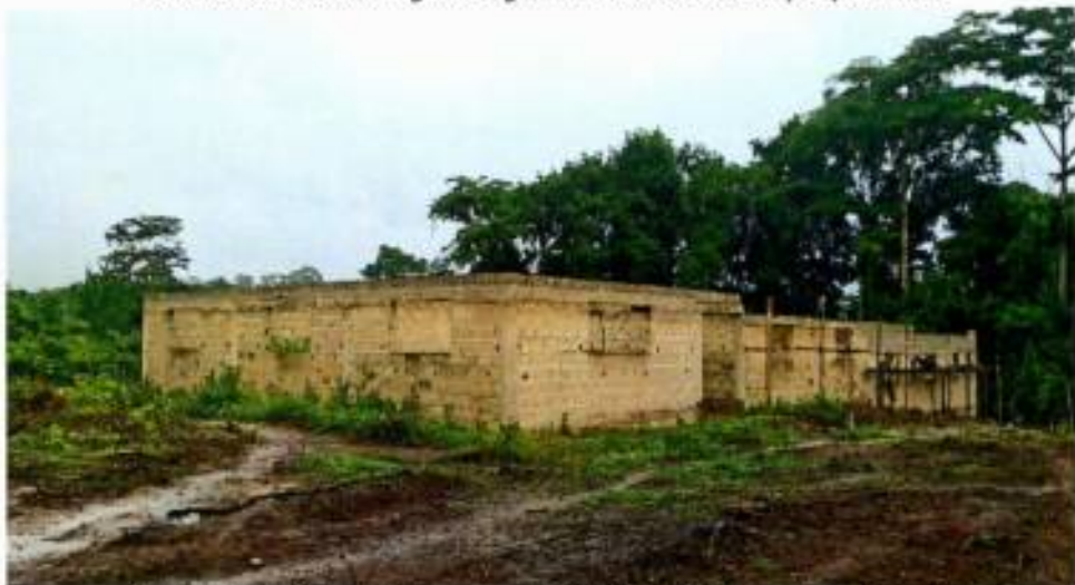
Construction of School Building – Cost: US$46,666.00 Gorkopa Town, Dist. #9; Blinnon Dist.: Contractor: Gleewill Liberia Limited
