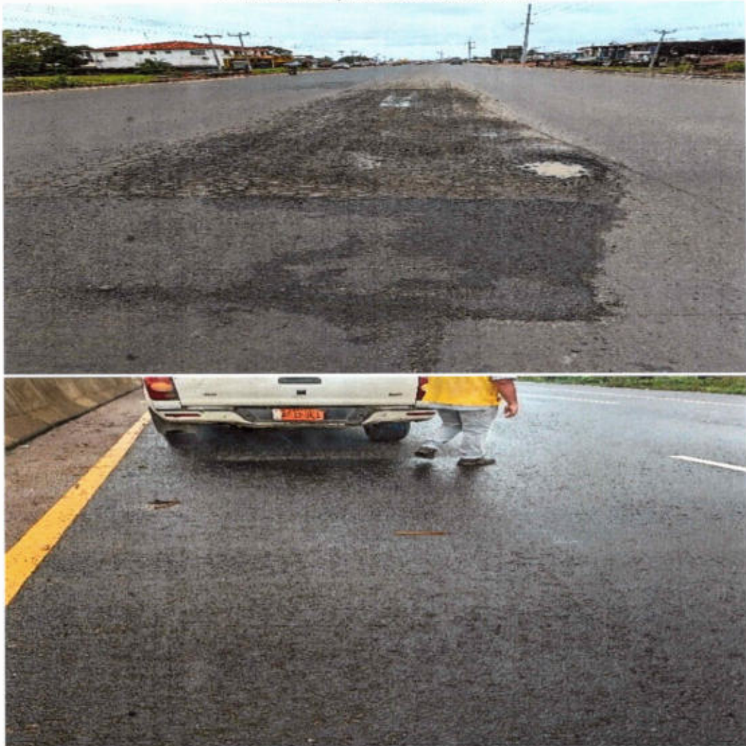
GAC Photo 1c: Showing Non-compliance with contract specifications (Depression/Settlement)
