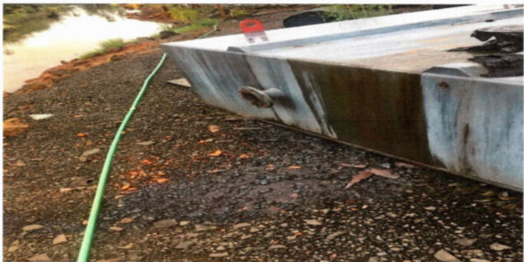
GAC Photo 3b: Showing no evidence that the drainage system was fitted with oil and grease interceptors
