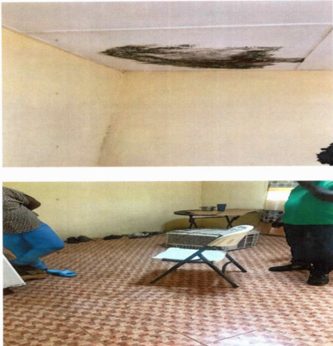
GAC Photo 2: Showing leakages, grass and the bushier areas inside the Project Camp
