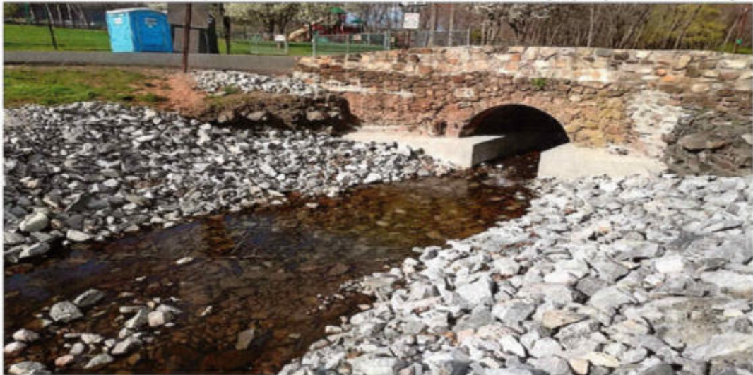
Photo 1a: Non-compliance with contract specifications (Riprap Protections)
