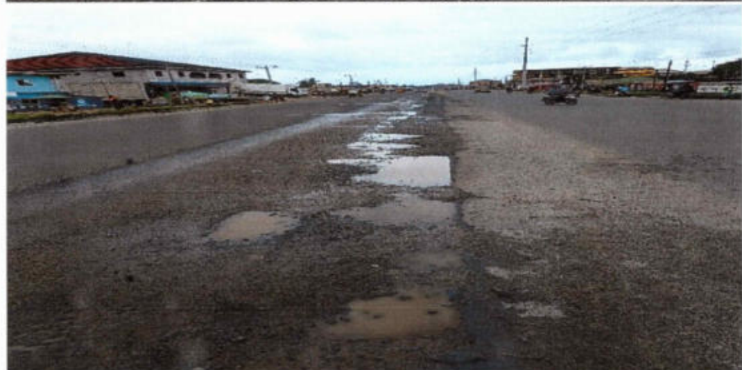
GAC Photo 1d: Showing Non-compliance with contract specifications (Cracks/Damage to Asphalt Binding Course)
