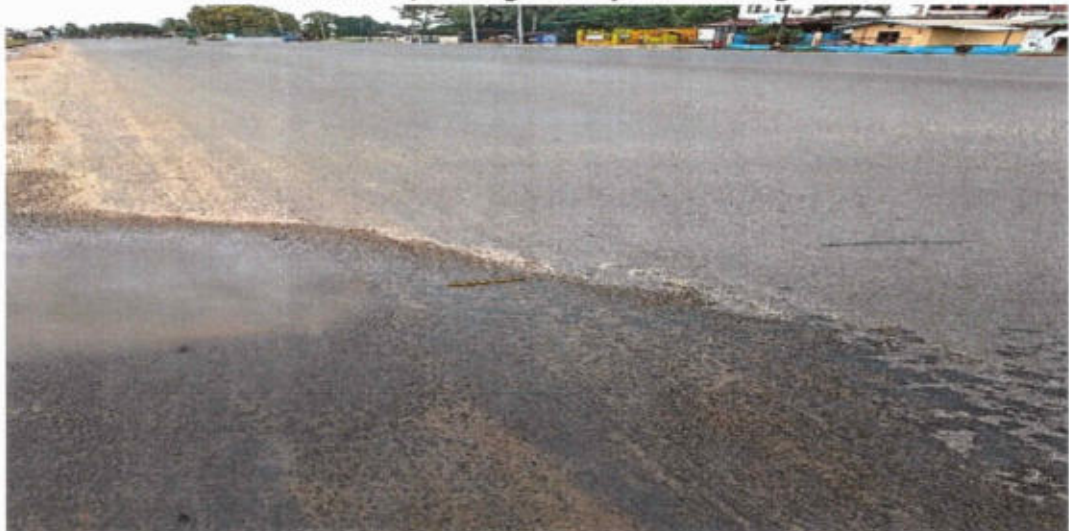
Photo 1d: Cracks/Damage to Asphalt Binding Course
