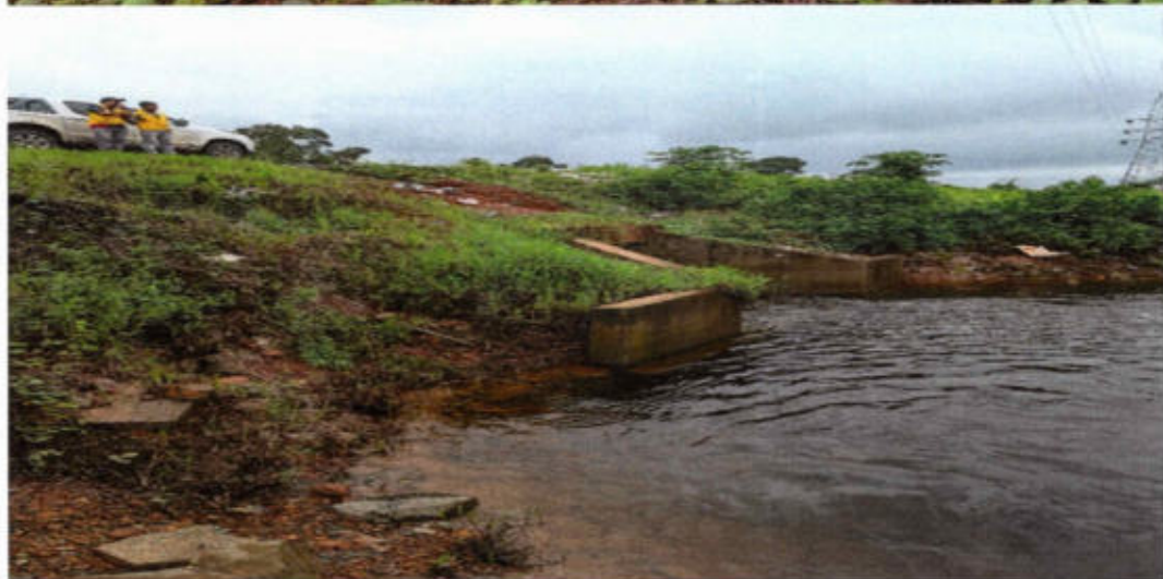
GAC Photo 1b: Showing Non-compliance with contract specifications (erosion around RCPs)
