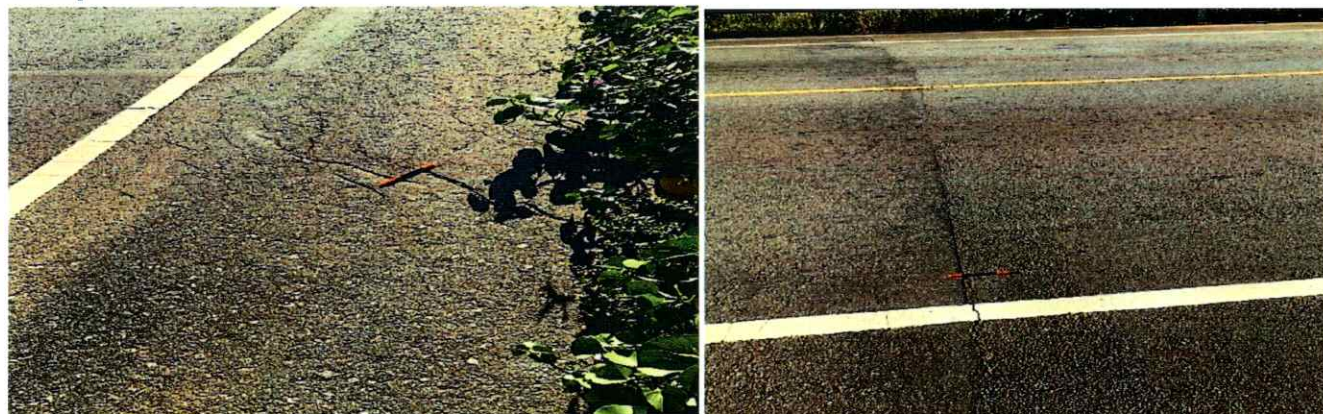
GAC Photo 5: Showing Unrepaired Crack on Asphalt along the Gbarnga to Ganta-Guinea Border Road Corridor in Lot 2
