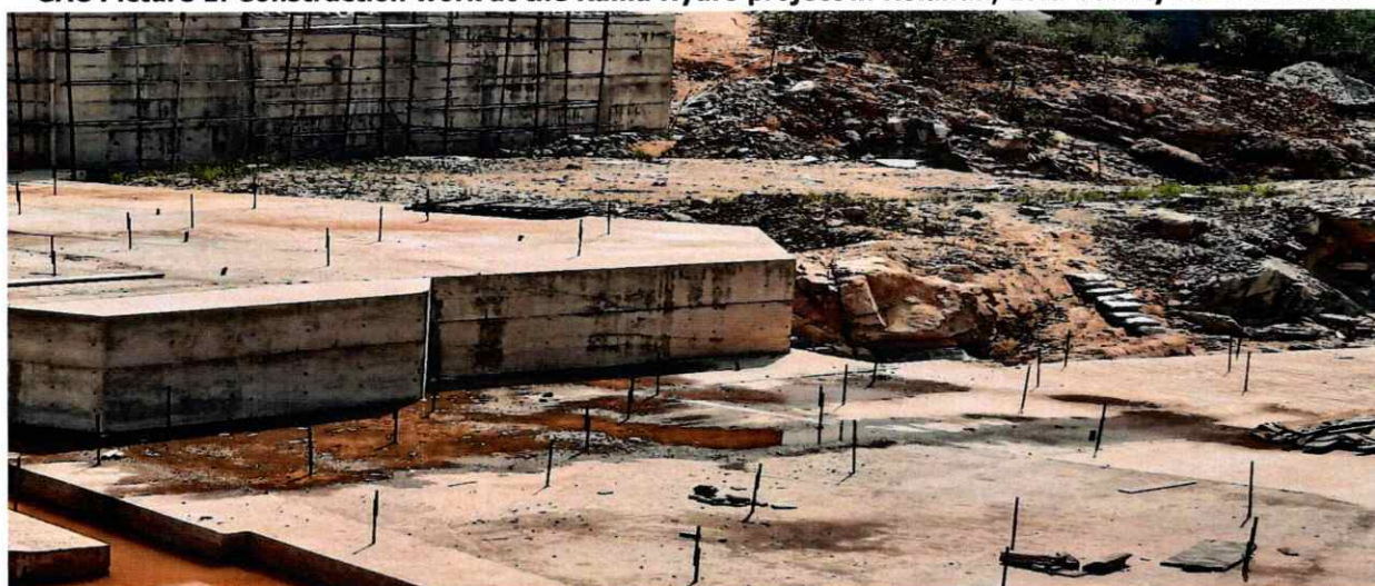
GAC Picture 2: Construction work at the Kaiha Hydro project in Lofa County
