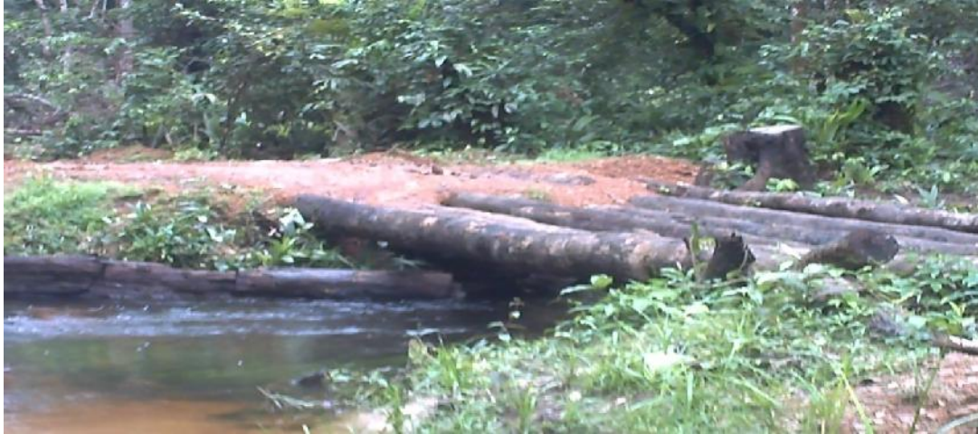
Figure 3: The end of the rehabilitation work at Wheasaye Town which started from Nyonbeh Town along the main high way from Buchanan leading to Sinoe County. The project did not cover the stretch of road from this point to the commercial fishing town of Grand Kola along the Atlantic Ocean.
